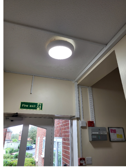
Lighting (Standard and Emergency Lights)
